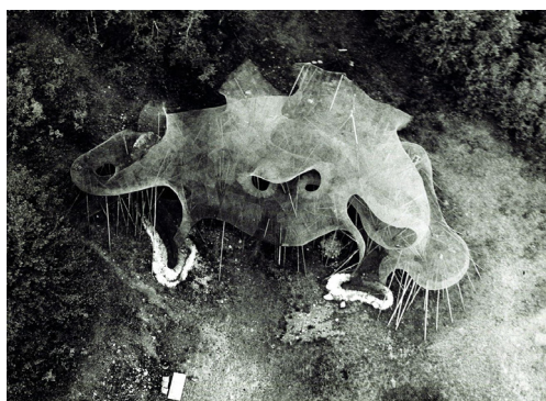
Figures 7,8 Vittorio Giorgini, Liberty community centre, Parkville, New York, 1976-77. Construction site photos. Retrieved December, 7, 2022 from < https://www.tribune.com/progettazione/architettura/2019/04/vittorio-giorgini-storia-italia/ >
